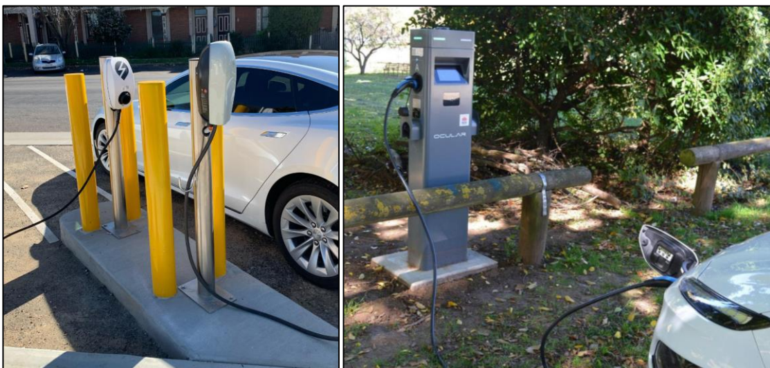
Bathurst Regional Council – Level 2 destination charging (‘wall mount’ left, dual port right)
