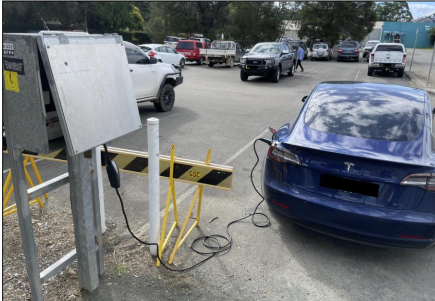
Gloucester Public Car Park – Level 1 Charging
